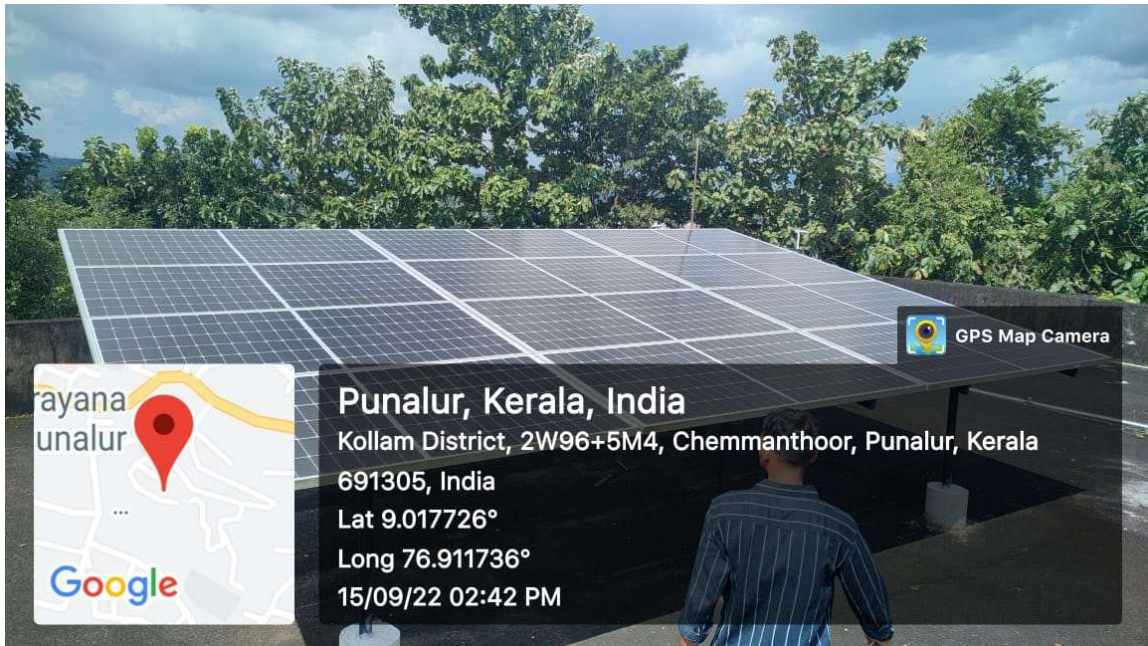
Image showing 5.2 kWh Solar Panel fitted on the roof of the Administrative building.
