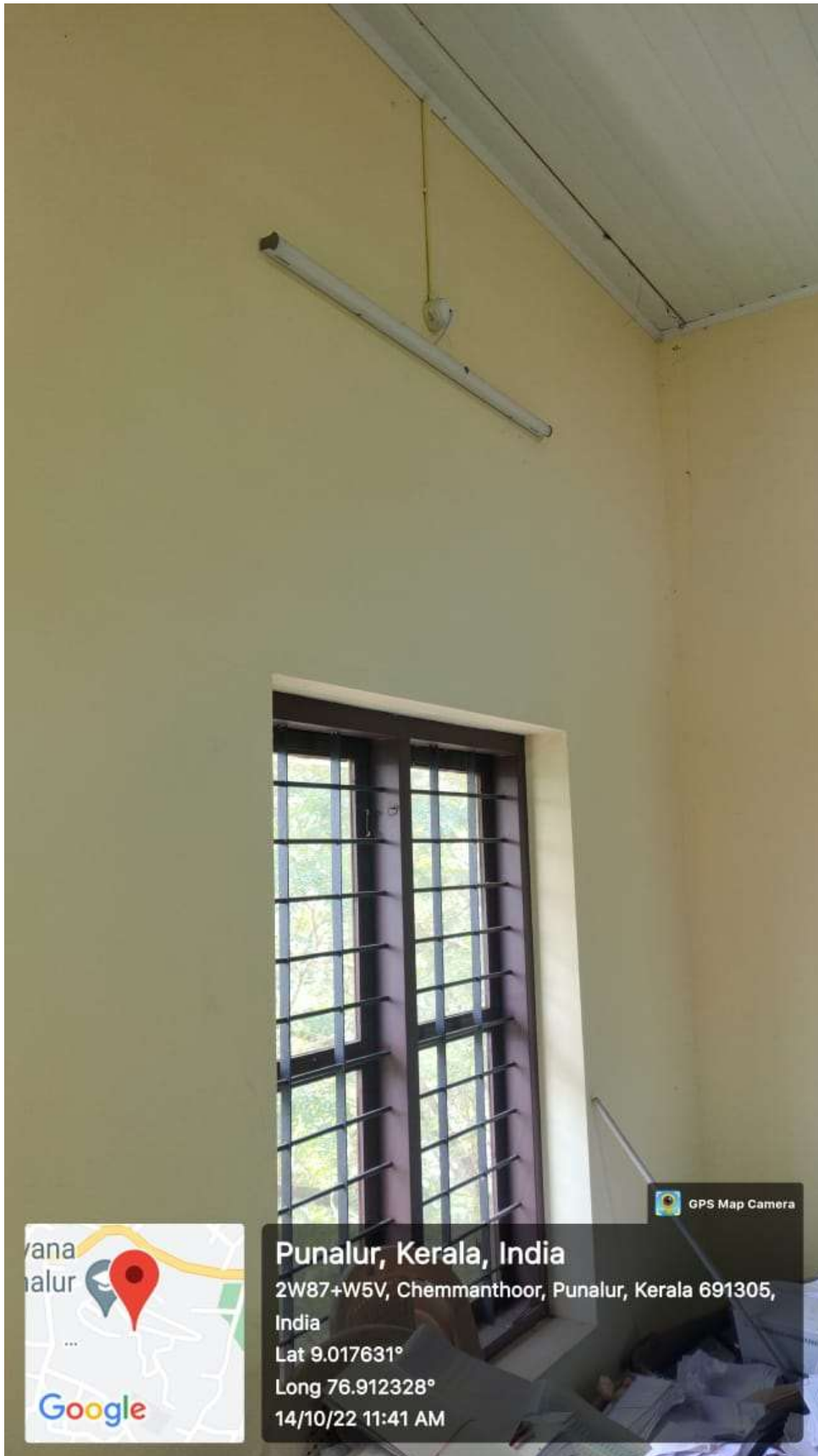
Energy saving LED Tube lamp in the Examination cell.
