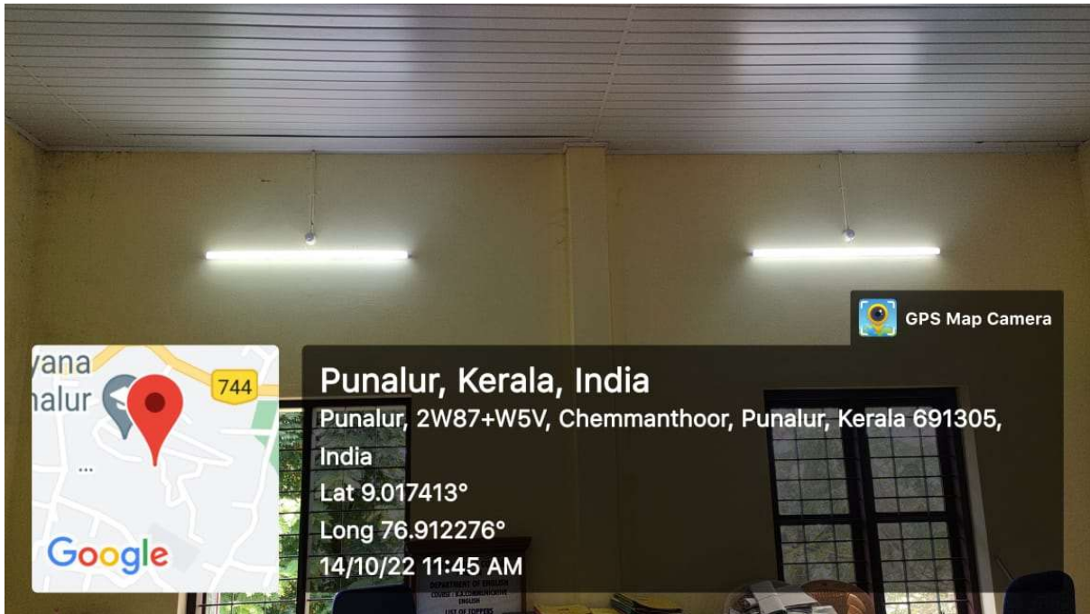
Energy saving LED Tube lamps in the IT Room.
