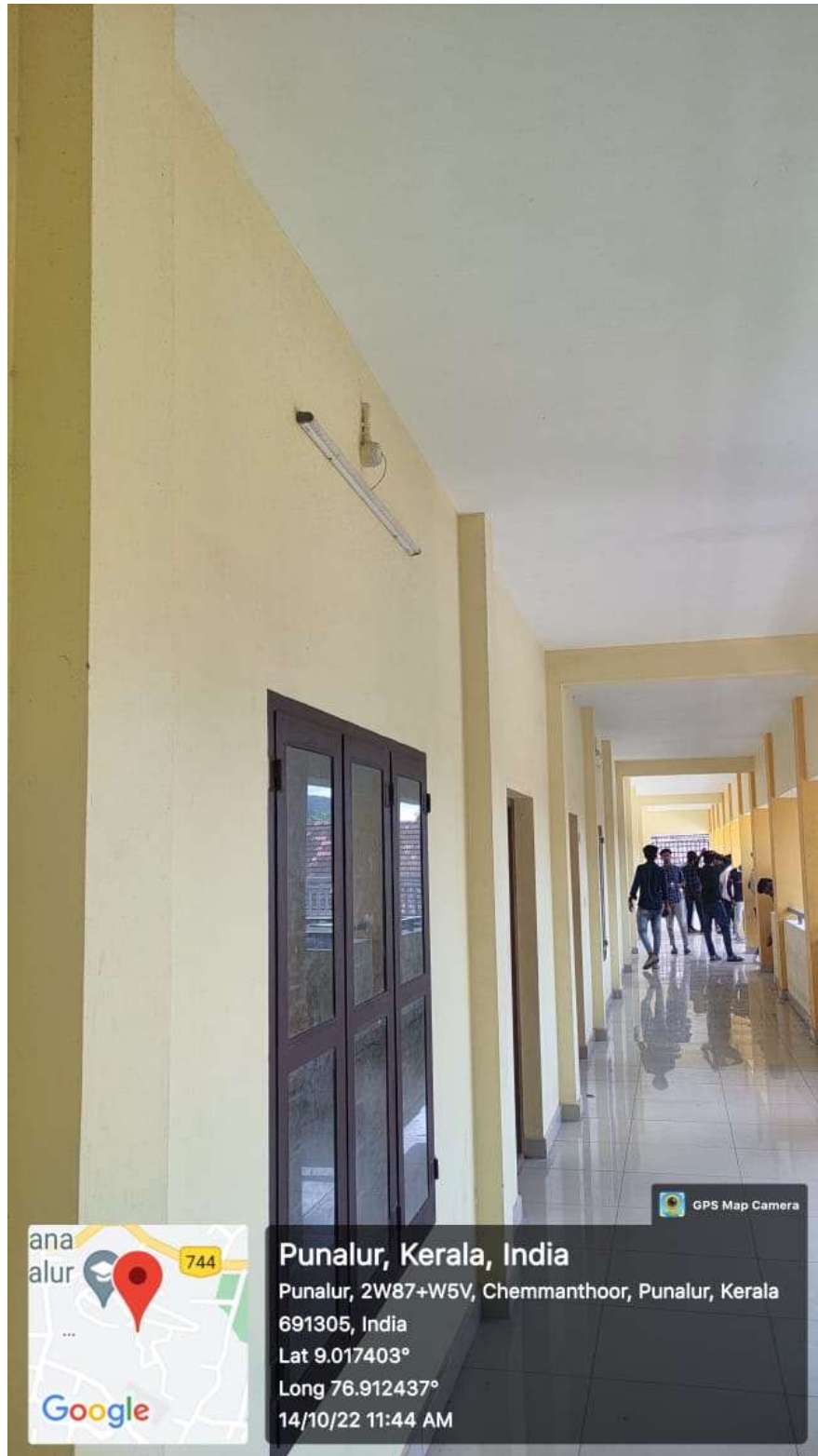
Energy saving LED Tube lamp in the First Floor Verandah.
