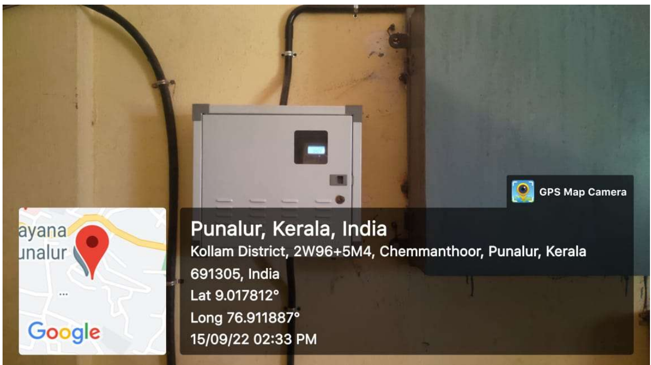
Bi-Directional Energy meter showing Solar Power Plant feed to the grid.
