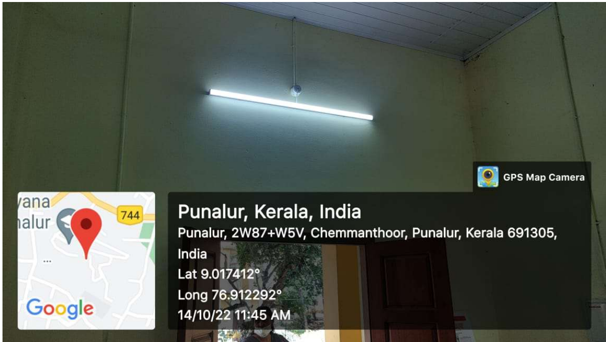
Energy saving LED Tube lamp in the Main-block classroom.
